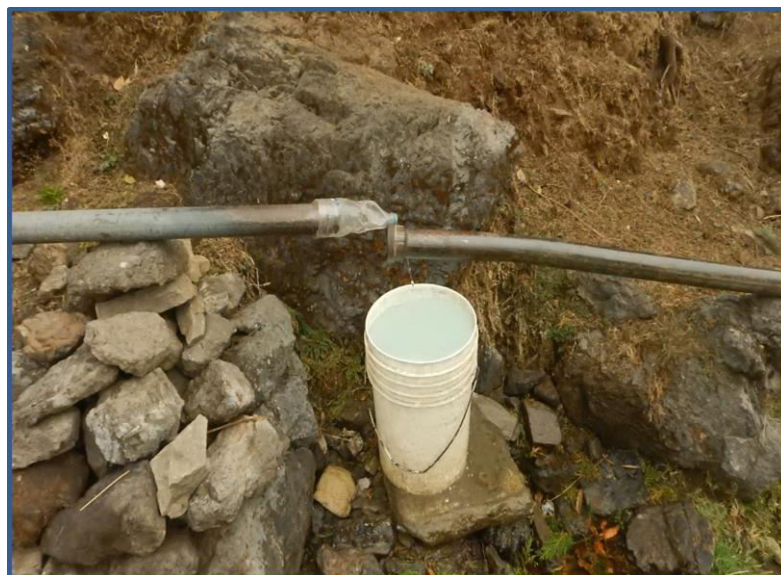
Fig. 7- Broken pipeline carrying spring water from the
